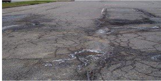
Fig 8: Effect of Rain on Pavement Design
