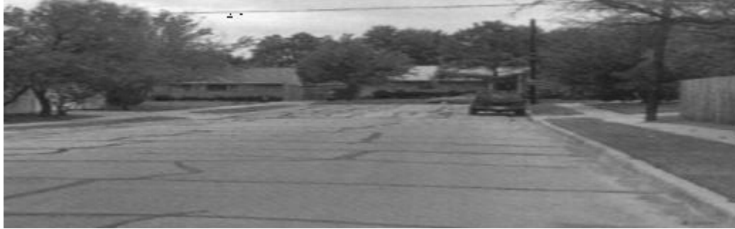
Fig.7: Swelling in Road Pavements
