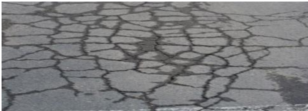
Fig.1: Alligator Cracks Formed in Flexible Pavements
