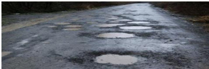
Fig.5: Potholes in Pavement
